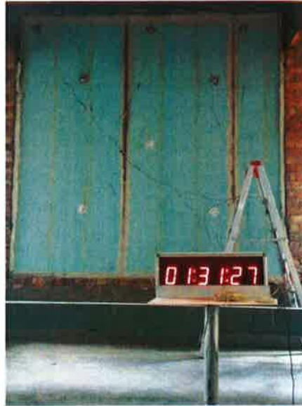
Unexposed face after the test
