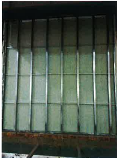
Inner structure of installation
